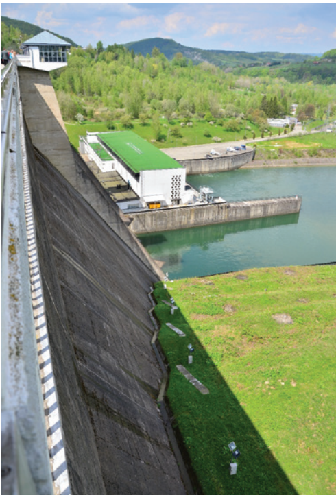
Fig. 1. Water reservoir in the municipality of Rutwica, zachodniopomorskie voivodship (photo M. Szkaradkiewicz)
